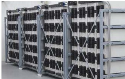
Energy Storage System
